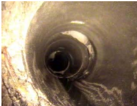
Figure 68 – (Photo 8) Joint décalé moyen
