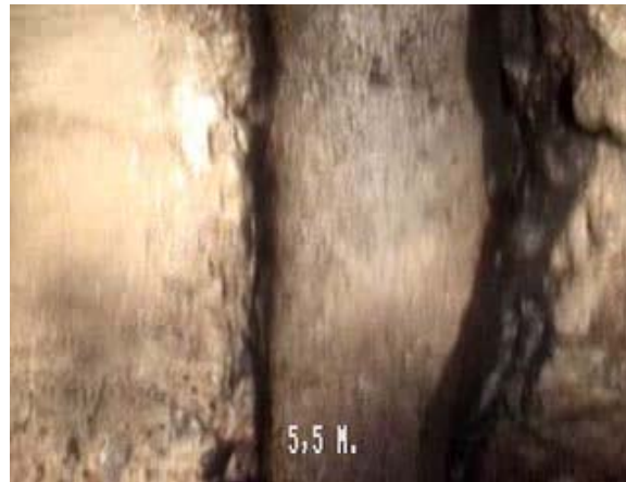
Figure 69 – (Photo 1) Trou au joint
