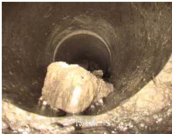
Figure 71 – (Photo 3) Raccordement obstrué
